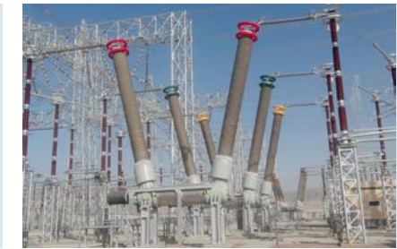
800 kV Circuit Breaker for Aksu Substation in Xingjiang
