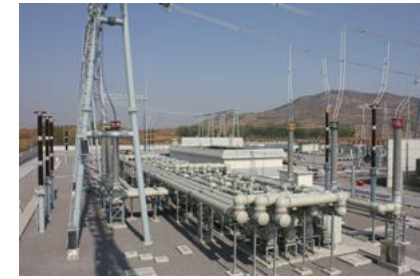
550 kV GIS for Xintai Substation
