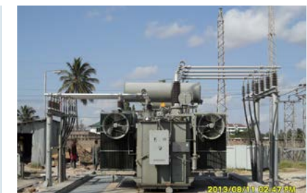
132/33/11kV Transformers for Ubungu Substation in Tanzania
