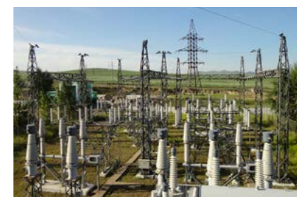
132 kV DMP Substation for Mongolia
