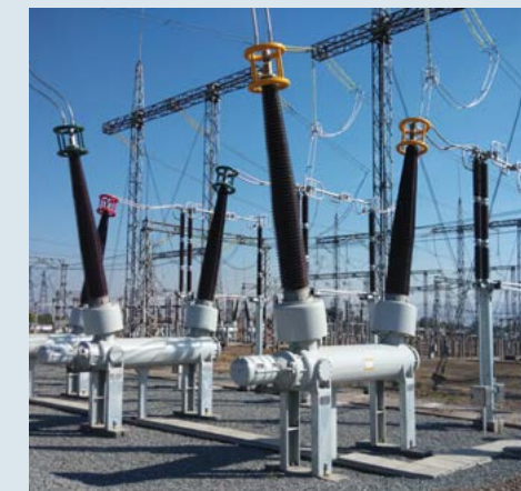
550kV Circuit Breaker
