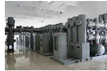
252 kV GIS for Mushan Substation in Shandong
