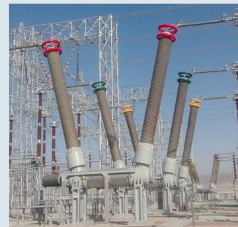
800 kV Circuit Breaker
