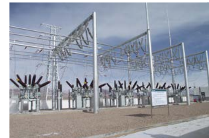
126 kV HGIS for Qinghai PV Substation
