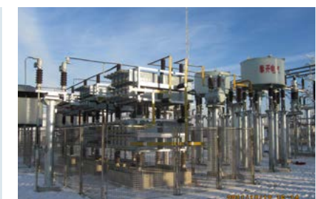
SVG for Guyang Substation in Inner Mongolia
