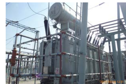
220 kV Transformer for Baotou Substation in Inner Mongolia
