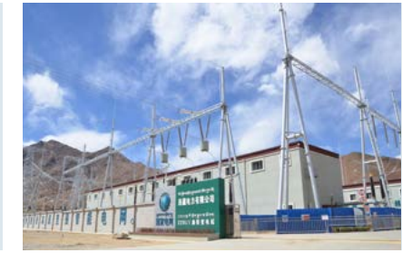
252 kV GIS for Quge Substation in Tibet
