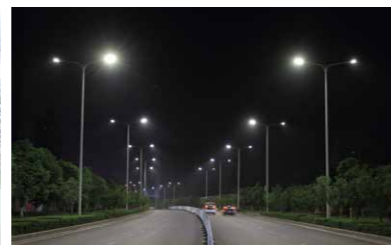
Intelligent Lighting on North Aixihu Road, Nanchang, Jiangxi province
